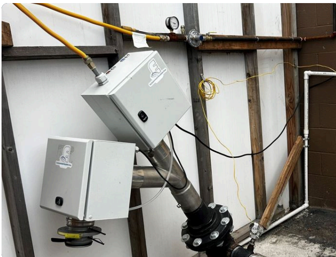
HETR™ wellhead with burner and control enclosures at Carson Plaza, Carson, California.
