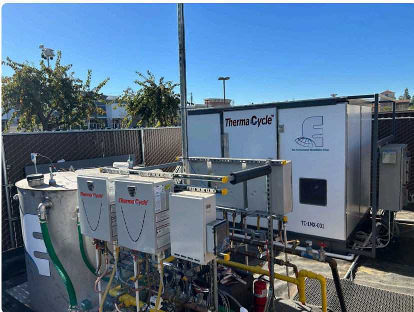
ThermaCycle® recirculation enclosure, heaters, controls and amendment tank, operating at an active commercial site in Southern California.
