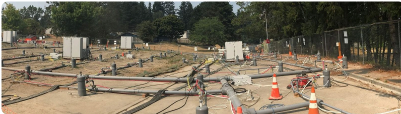
The 76-electrode ERH wellfield at the Jackson Park NEX Gas Station Leak Area.
