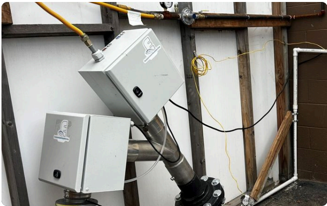
HETR™ wellhead with burner and control enclosures at Carson Plaza, Carson, California.
