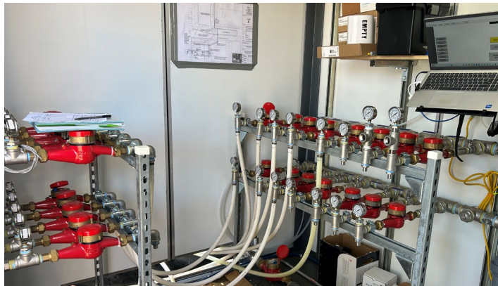
Wellfield distribution manifold — individual zone flow control, instrumentation, and inline dosing integration
