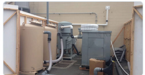
Vapor extraction and treatment system.
