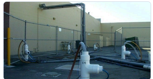
Thermal and vapor extraction wellheads.
