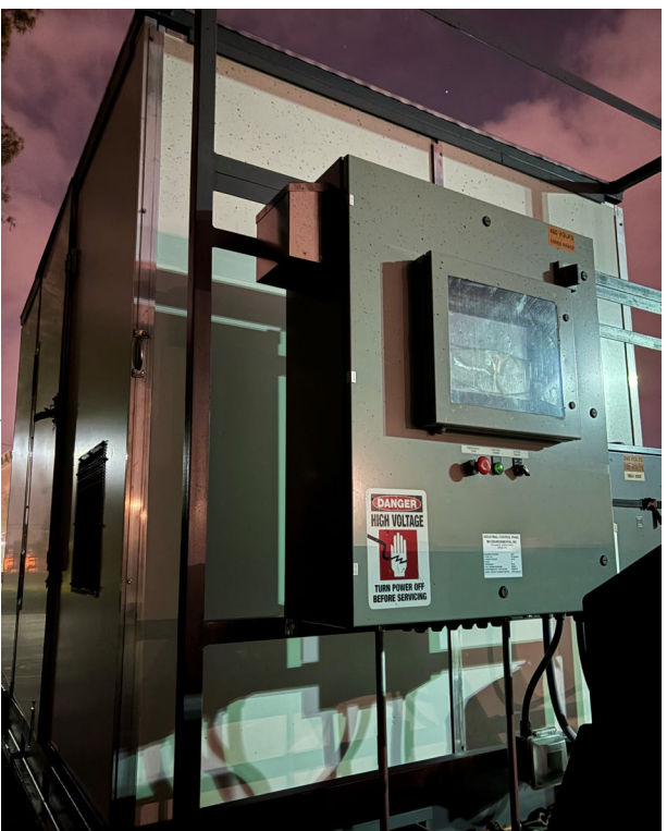
8.5 × 12 ft all-metal process enclosure, fully piped, wired, and factory-tested
