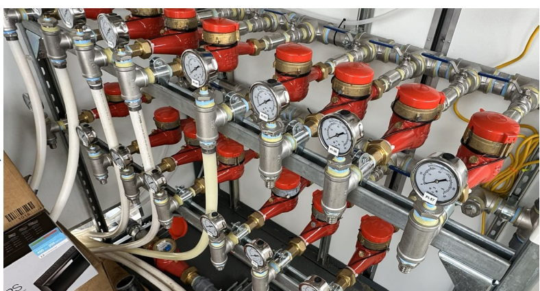
Manifolding Pre-plumbed “plug and play” injection and extraction manifolding with flow meters, inline sensors (Ph, temp, pressure, etc.)
