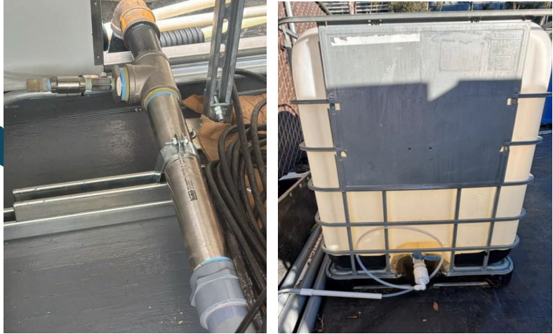
Integrated Dosing Static mixer — integrates multi-chemical dosing in-line with heated water pre-reinjection
